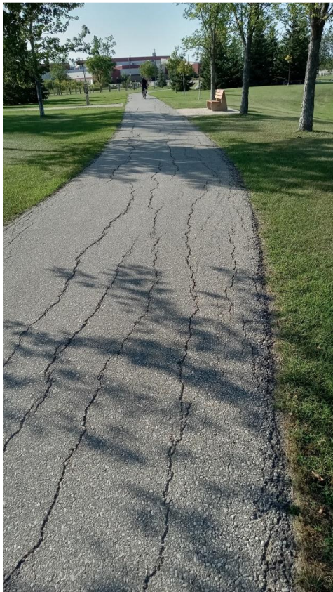
Photo: Linear cracks on the Creek Path. Frost jacking will open these to 30mm or more by late winter.
